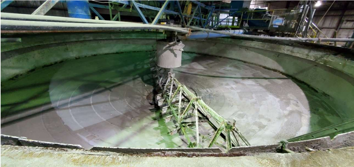
Figure 12.4 – Mill under maintenance (1)
